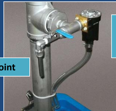
Temperature Control Valve and Drain
