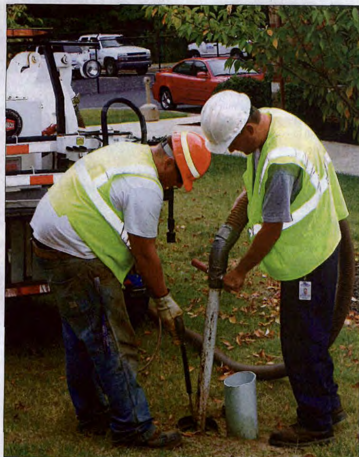
Forest Hill (left) and Glenn McCarty use the vacuum function on the valve exercising trailer to clean a valve box.
