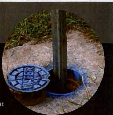
A valve key connected to the district's trailer-mounted valve maintenance system is turned to exercise a valve.
